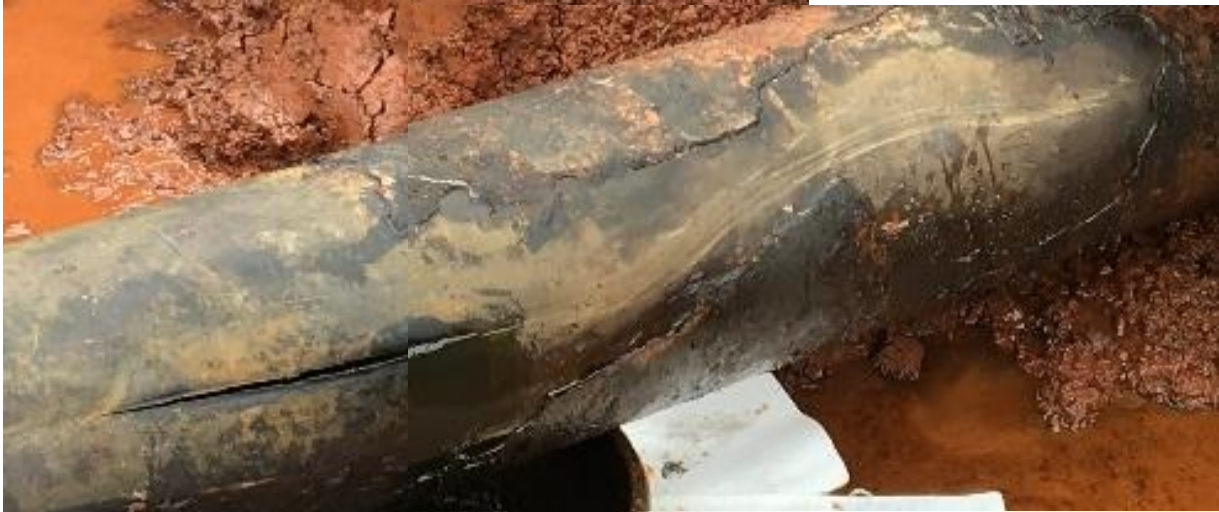
Figure 3: Previous Second Party Excavation Damage
