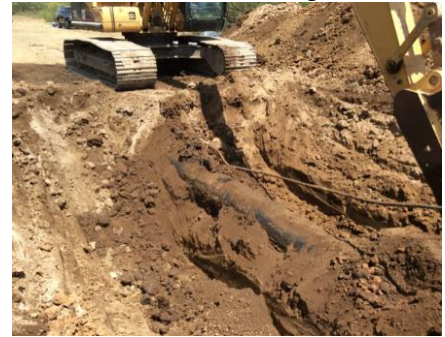
Figure 8: Conduit Veering Toward Pipe
