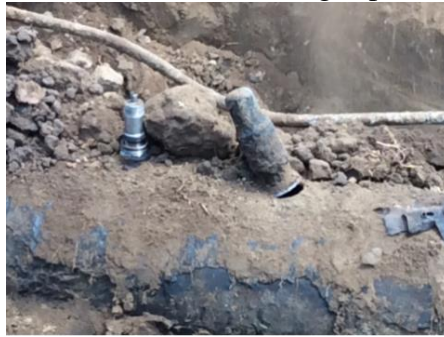
Figure 7: Excavation Damage to TOR
