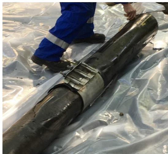
Figure 2 - Excavation Damage from Backhoe
