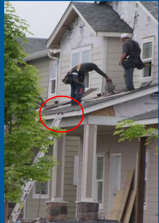
Improper ladder set-up (not 3 ft. above roof line)
